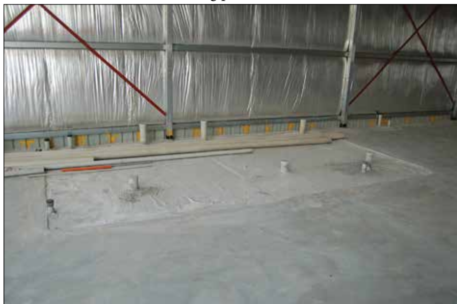
The site of the toilet block and kitchen with pipes peeking coyly through the concrete.
