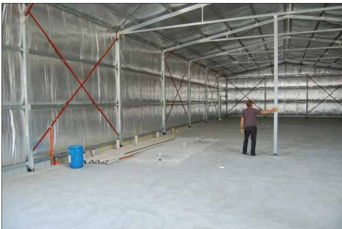
Nick Danielle poses by one of the support pillars to give some idea of the scale of our new club rooms building.
