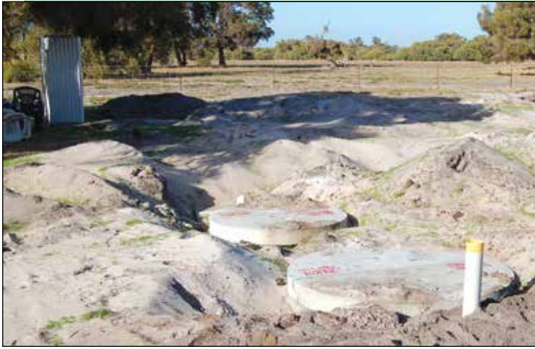
The septic tanks with the temporary facilities in the background
