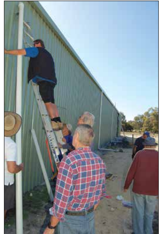
David Moir lifts the last of the north side downpipes into position with Steve Gilmour up the ladder ready to guide the top home. Others are Michael Broughton, Lindsay Hamersley holding the ladder, Brian Eyre, Thierry Michot and Ross Oxwell.
